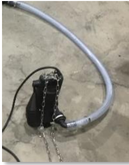
Connect One End of the Hose to The Pump
